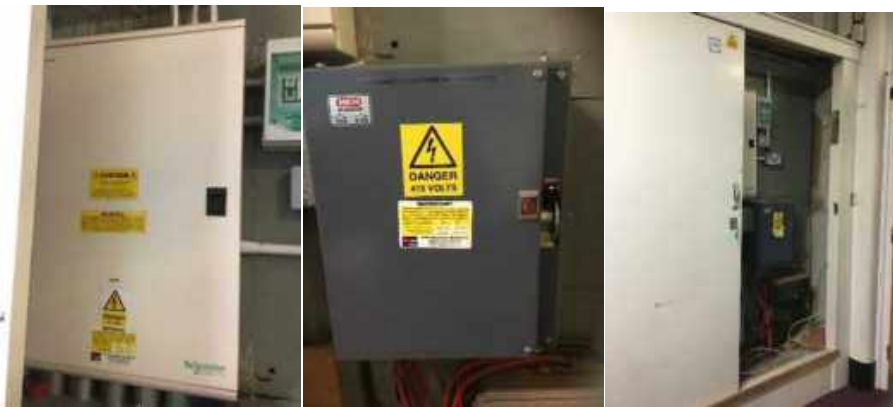
Electric isolation and meter, main school, link corridor, between reception and Year 3
